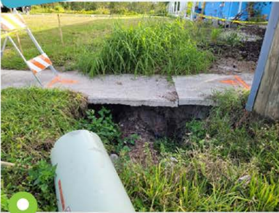
DAMAGED DRAINAGE OUTFALL PIPE ON GARDNER DRIVE
