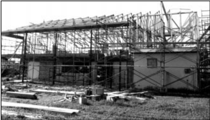
Figure 3-6 The owner of this floodprone house in south Florida decided to build a new frame second story on top of his masonry first story. The new second story is well above the BFE.
