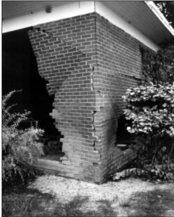
Figure 2-11 Moving water can cause walls to collapse, as illustrated by this riverine flood damage in Georgia.
