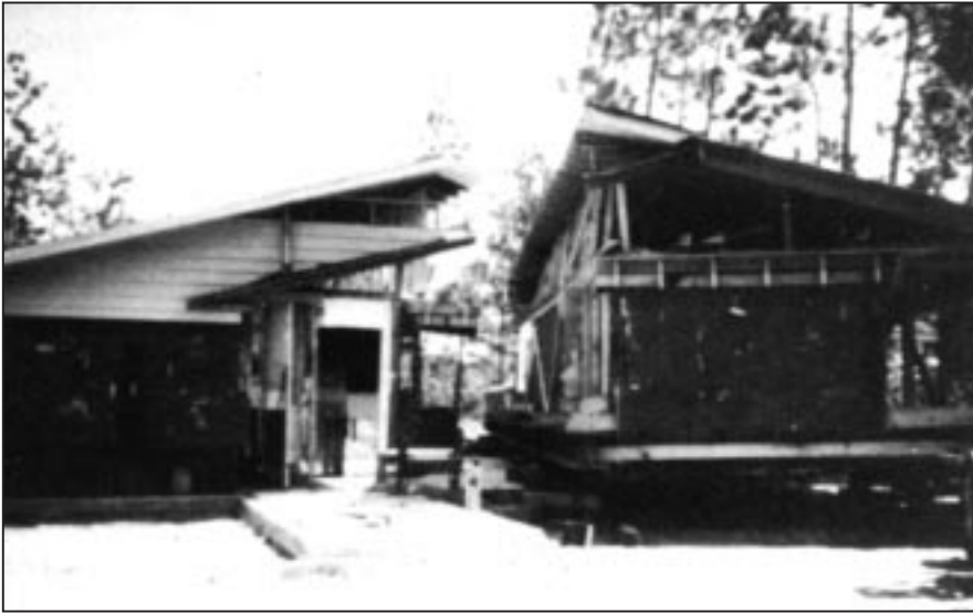
Figure 7-1 When a house is too large to be moved in one piece, it must be cut into sections that can be moved separately and then reassembled at the new site.
