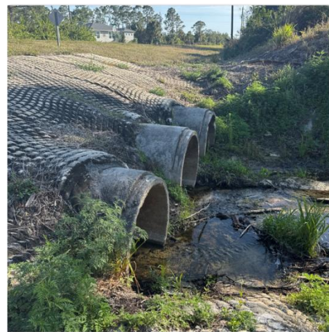
Figure 5: Site visit photo of large triple RCP crossing near Tropical Gulf Acres
