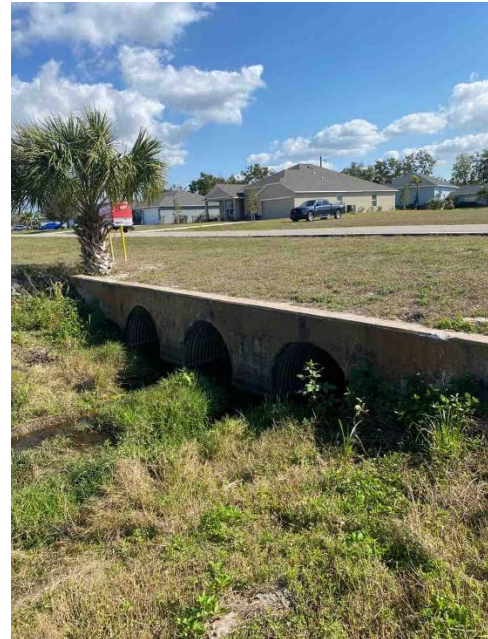
Figure 6: Site visit photo of large RCP culvert crossing in Burnt Store Village
